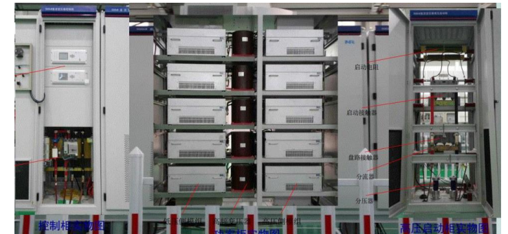
Hangzhou Dajiangdong DC Distribution Network Demonstration Project \pm 10\text{kV}/\pm 375\text{V}/500\text{kW} SST
