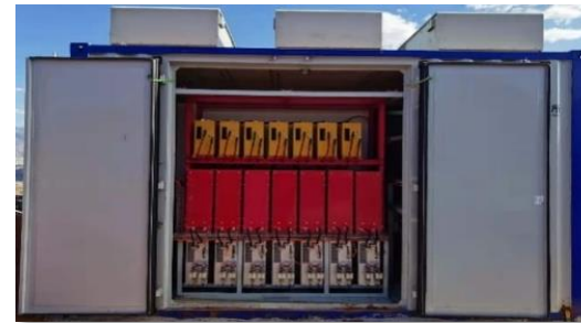
IEECAS ±30kV/1MW PV DC Step-up Converter
