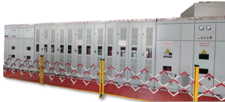
Wujiang MVDC/LVDC Power Distribution System Demonstration Project \pm 10\text{kV}/750\text{V} 2MW SST
